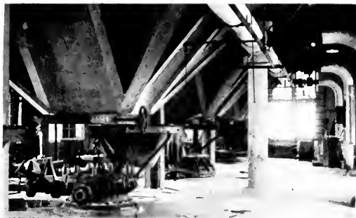
Part of Charging Floor, Digester House. Note Bottom of Concrete Chip Bins and Steel Filling Funnel.
